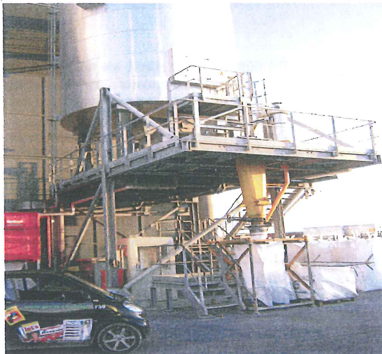
SILO FOR COLLECTING APCr IN BAGS
